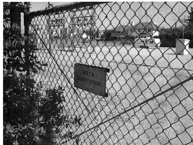
11. View of PG&E substation.
